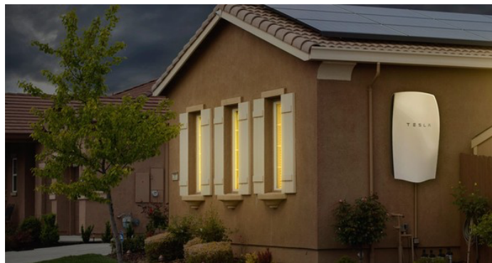
Figure 2. A Tesla Powerwall installation (Tesla, n.d.)
